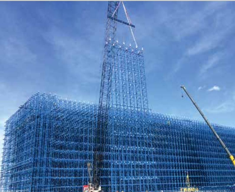
The logistically efficient, clad-rack structures are not yet as common in the US as they are in Europe.
