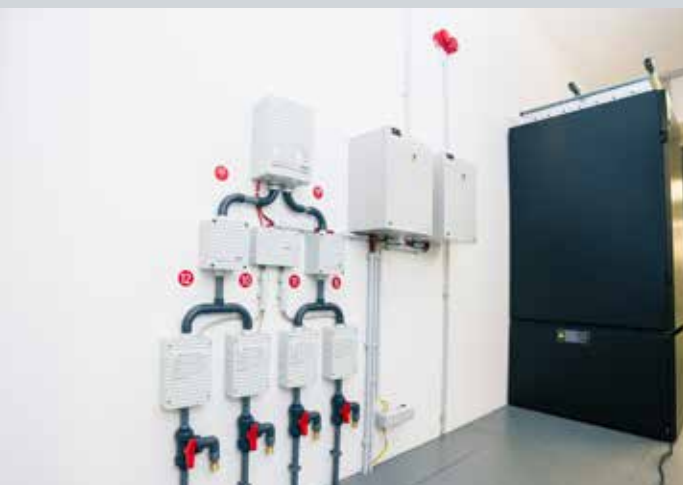
Air sampling smoke detector
