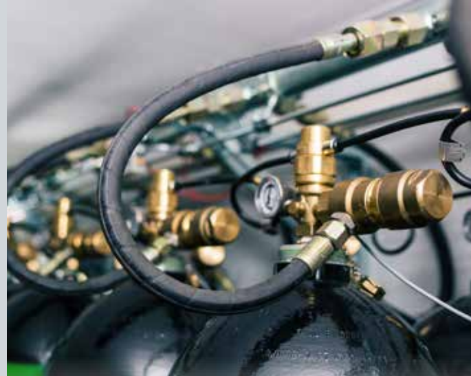
Flow regulators were attached to the extinguishing agent cylinders in order to minimise pressure spikes at the start of the extinguishing process.
